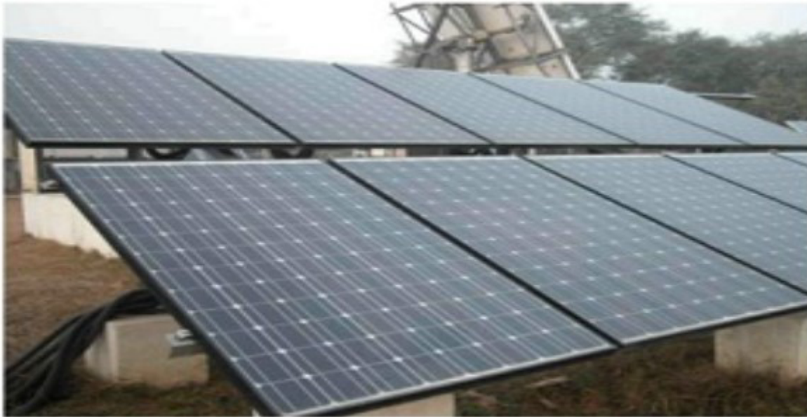
Figure 1 mc-Si PV module installed at NISE
